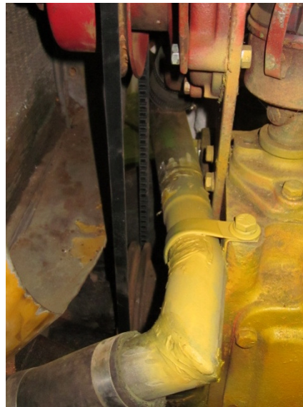
Crossing in front and into the radiator
